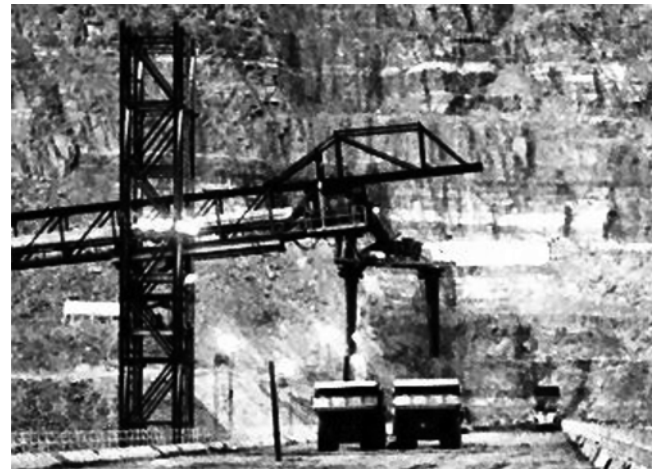
Fig. 6.7—Discharge conveyor that allows uninterrupted loading of RCC into adjacent trucks, Upper Stillwater Dam, UT. (Photo courtesy of U.S Bureau of Reclamation, 1986.)
