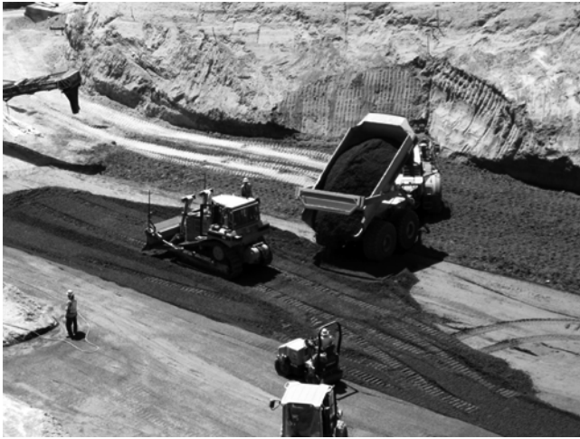
Fig. 6.8—Dumping fresh RCC onto previously placed and spread, uncompact lift, Deimer Dam Modification. (Photo courtesy of MWH Global, 2007.)
