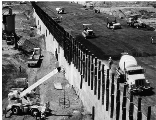
Fig. 6.17—Precast panels for upstream face of Willow Creek Dam, OR. (Photo courtesy of U.S. Army Corps of Engineers, 1982.)
