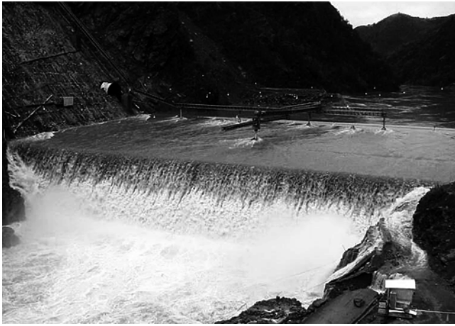
Fig. 1.11—Le Presa Ralco Dam, Chile, overtopping during construction. (Photo courtesy of B. Forbes and E. Warren, 2003).
