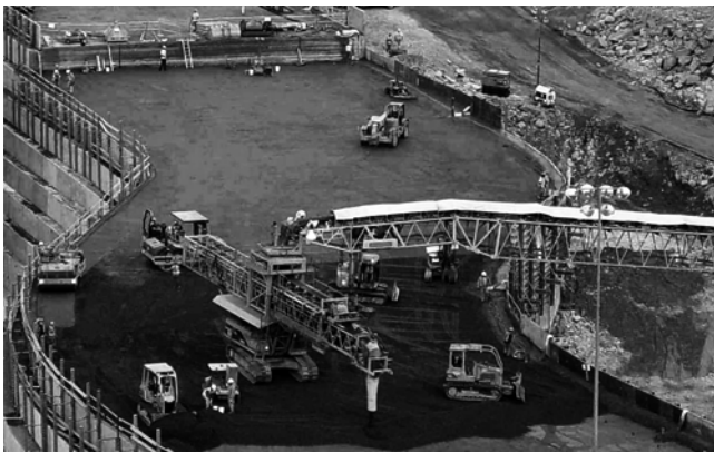
Fig. 6.5—RCC placed on dam body with crawler-mounted conveyor on dam surface, Saluda Replacement Dam, SC. (Photo courtesy of Barnard Construction, 2004.)
