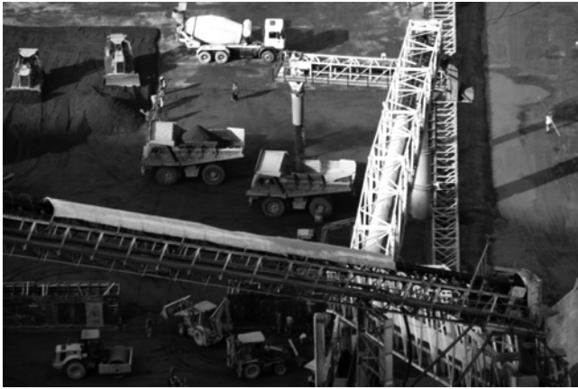
Fig. 6.1—Transporting RCC by conveyor discharging to waiting end dump trucks on lift surface, Al Wehda Dam, Hashemite Kingdom of Jordan. (Photo courtesy of Edward Warren, Water Power and Dam Construction, 2009.)
