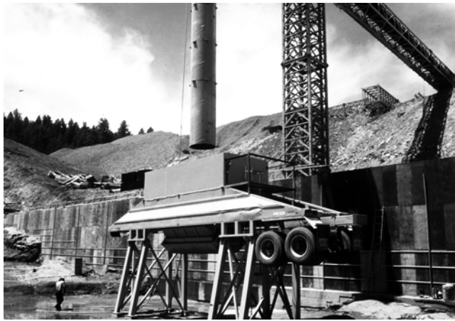
Fig. 6.2—Partial conveyor system to hopper on dam.
