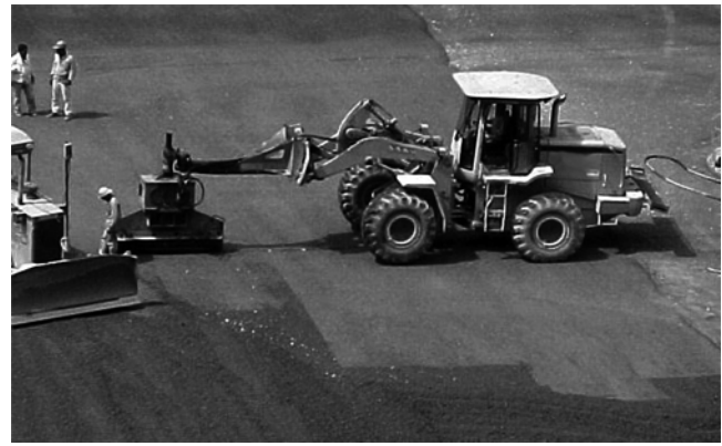
Fig. 6.11—Crack inducers inserted by vibrating plate on front end loader, Miel I Dam, Colombia. (Photo courtesy of INGETEC S.A., 2002.)
