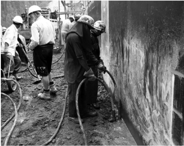
Fig. 6.14—GERCC: consolidating GERCC with hand-held immersion vibrators at upstream formed facing, Kinta Dam, Malaysia (Forbes 2008).
