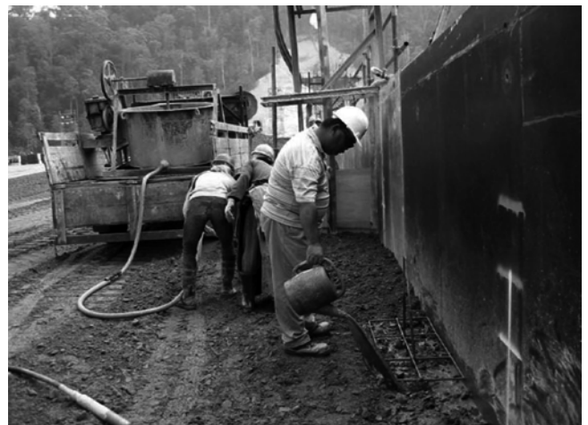
Fig. 6.13—GERCC: adding grout onto surface of unconsolidated RCC along upstream form, Kinta Dam, Malaysia (Forbes 2008).
