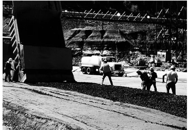
Fig. 6.9—RCC dumped and spread with controlled tailgate in 16 in. (400 mm) loose layers prior to compaction. (Photo courtesy of U.S Bureau of Reclamation, 1986.)
