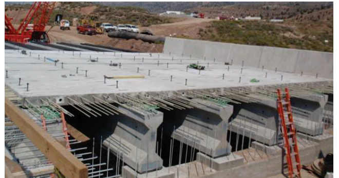
Fig. 3.2d—Emma Park Bridge deck panel with GFRP reinforcing bars, top and bottom mat.
