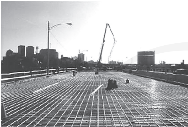
Fig. 3.2b—GFRP bars used in the redecking of Dayton, OH, Salem Avenue Bridge in 1999.
